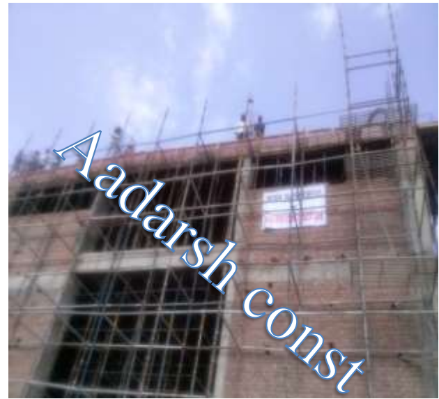
Pouring of Concrete in Terrace Slab of Commercial Building at HSIDC, Sector-35, Gurgaon
