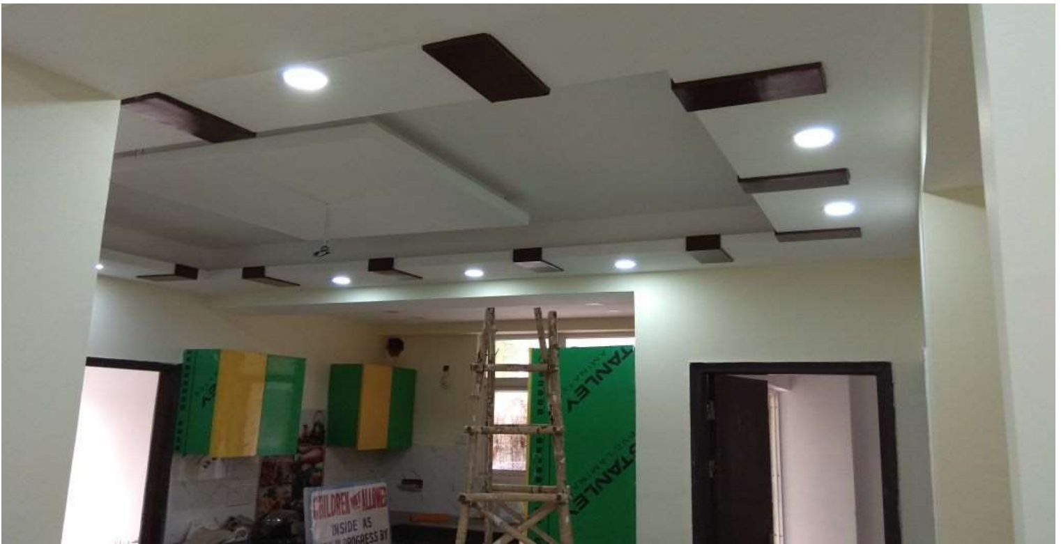
Broad View of Dining Room and Kitchen , work in Progress approaching completion
