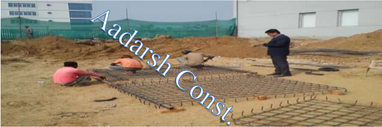
Construction of RCC Building HALL of FSTC at the time of FOUNDATION
