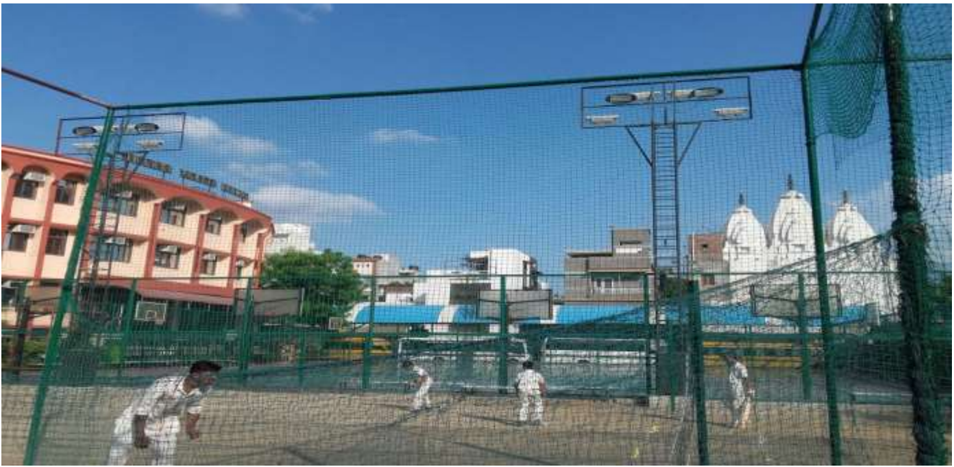
Flood Light Installation and making of cricket Pitch at Bharti Public School
