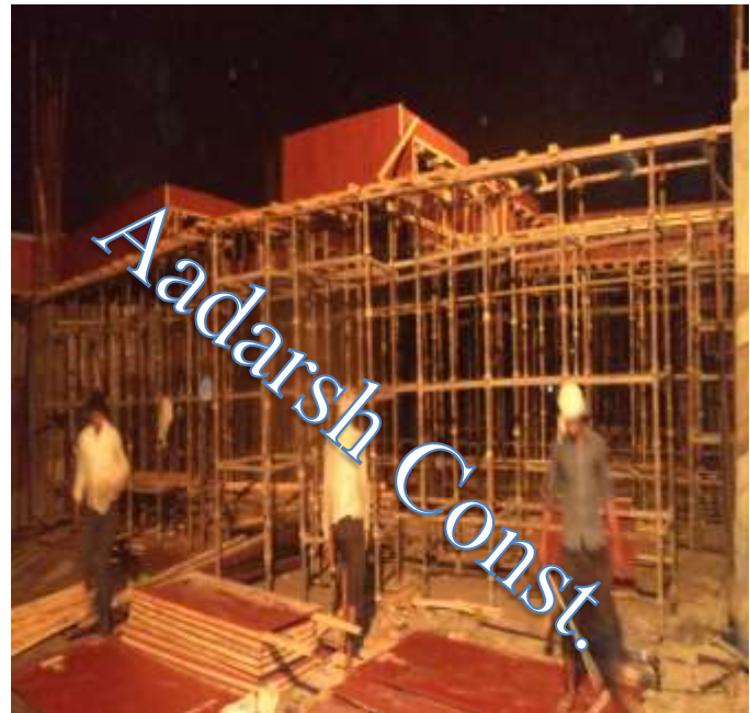
Centering & Shuttering of Terrace Slab of Commercial Building at HSIDC, Sector-35, Gurgaon
