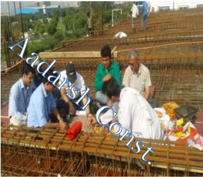
Pooja before casting of Terrace Slab of Commercial Building at HSIDC, Sector-35, Gurgaon
