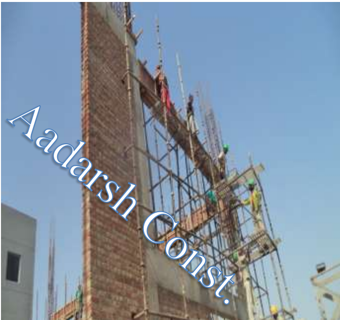
Casting of 2 nd Floor Beam of Commercial Building at HSIDC, Sector-35, Gurgaon
